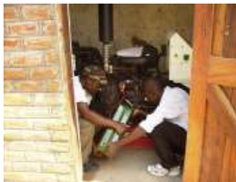
Fueling the generator
